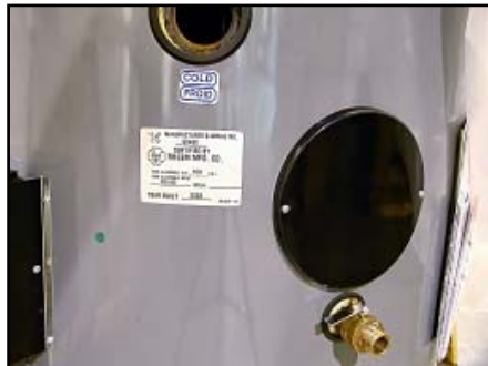
Exterior ASME plate located next to hand hole cleanout pan.
