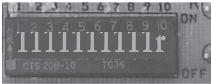
(This board is located in the blower section)
