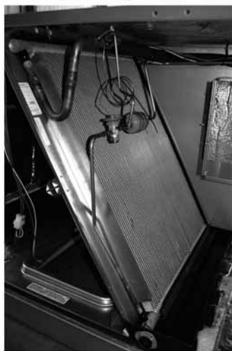
Evaporator Coil/Filter Access
