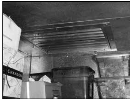
Inside view of an installed walk-in cooler
