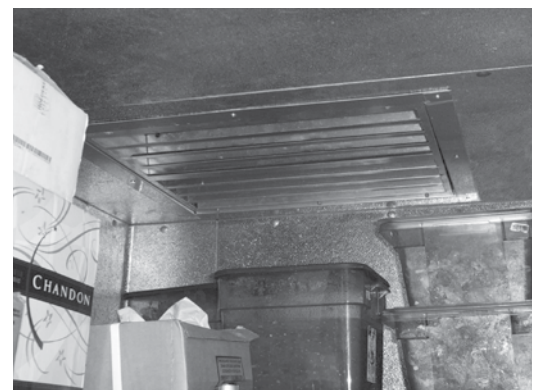
Inside view of an installed walk-in cooler.
