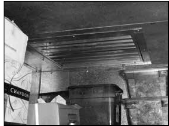
Inside view of an installed walk-in cooler.
