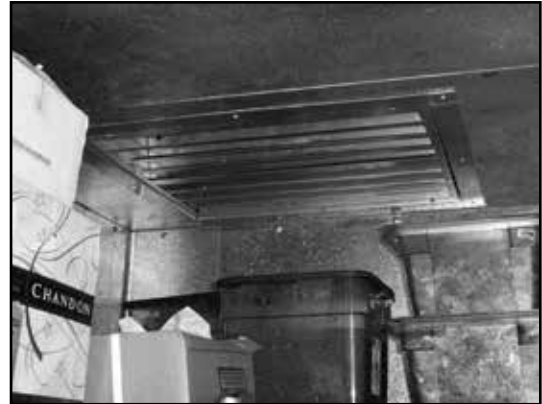
Inside view of an installed walk-in cooler.
