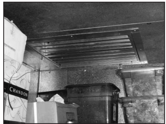
Inside view of an installed walk-in cooler.
